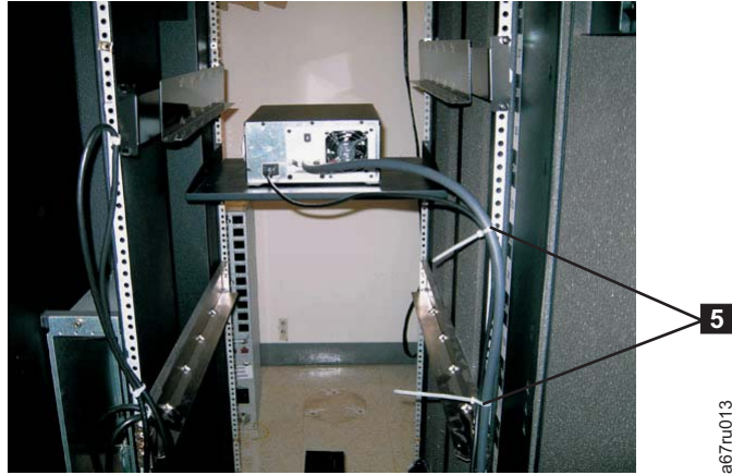
Figure D-2. Rear view of shelf with cables attached to rack rails with tie wraps
