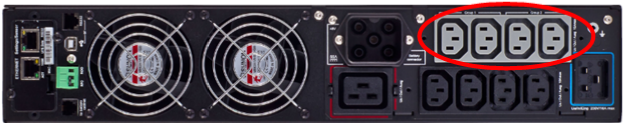
Figure 80: Programmable outlets for non-critical hardware
