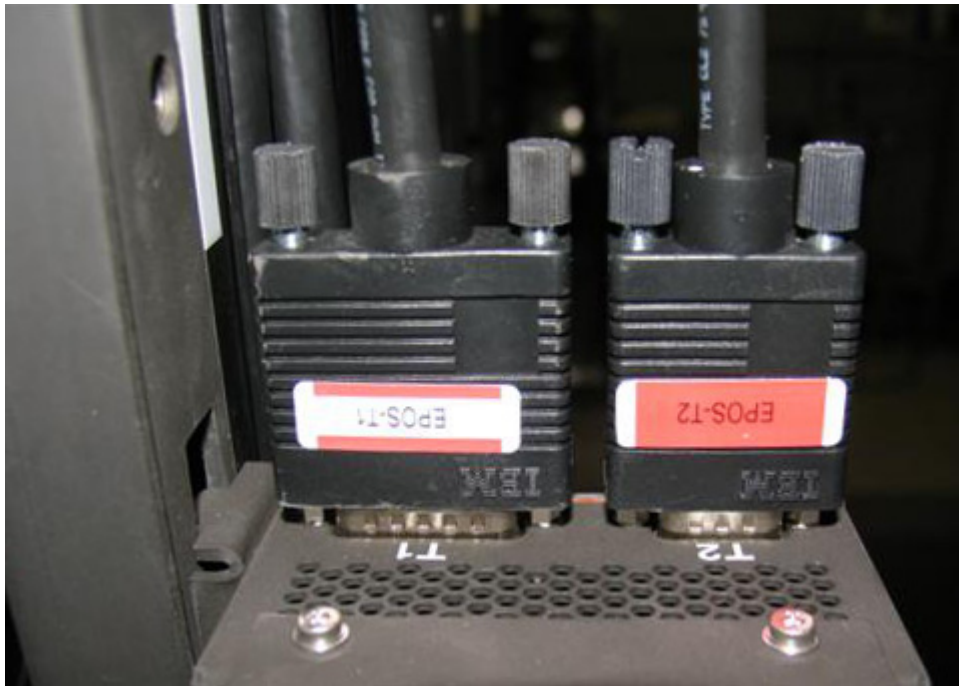
Figure 15 UEPO Cables Plugged into UEPO Panel
