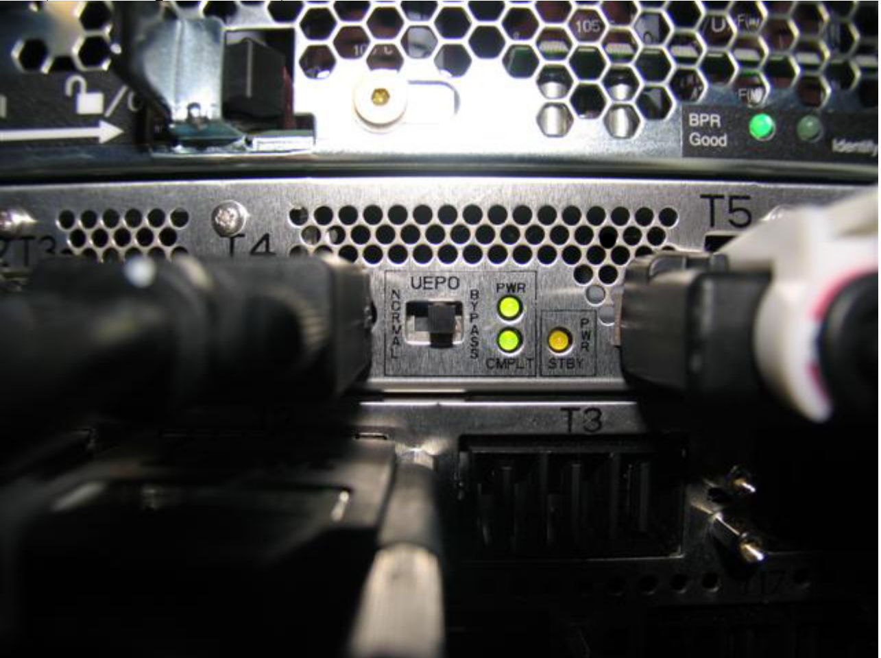
Figure 11 BPCH UEPO Bypass Switch shown in desired BYPASS position (moved to the right)
