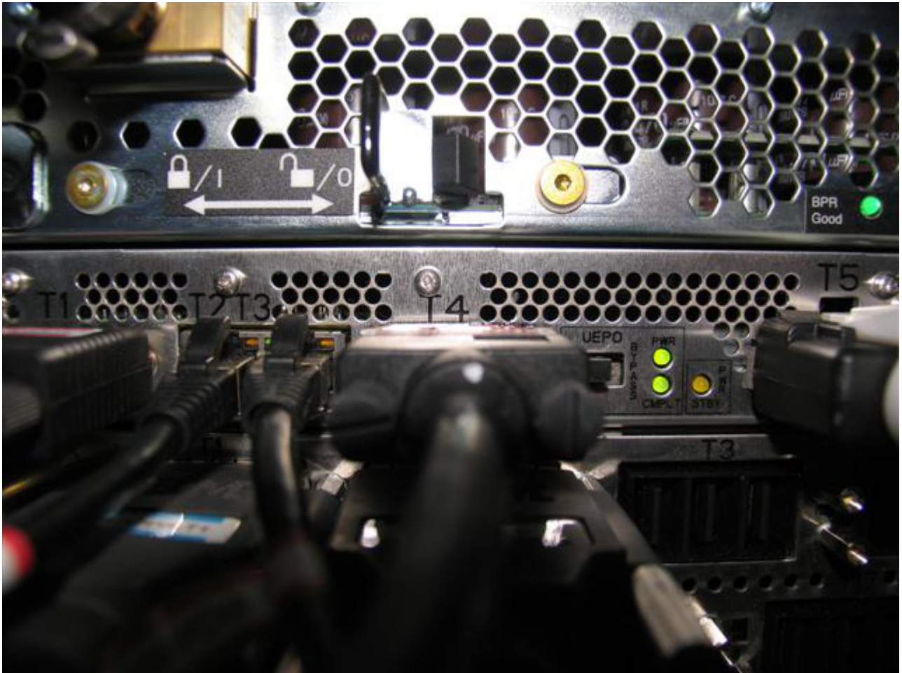
Figure 14 UEPO Cable Plugged into BPCH
