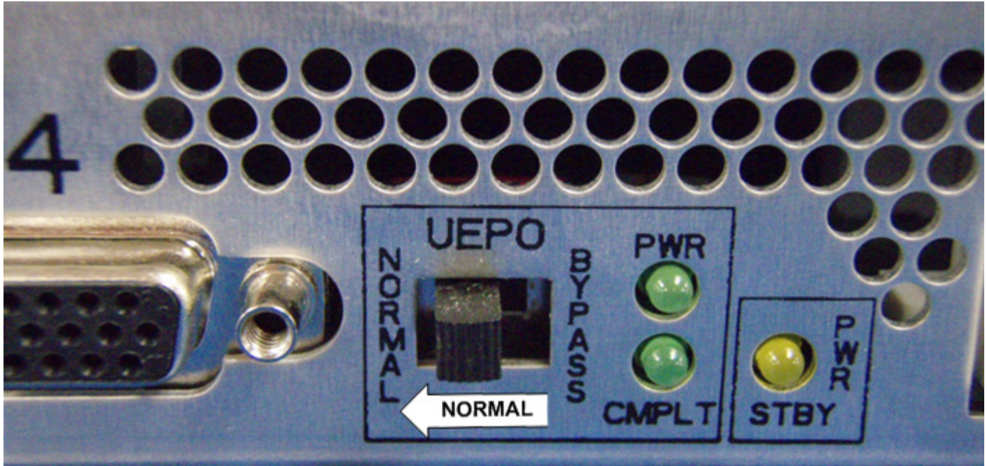
Figure 16 BPCH UEPO Bypass Switch shown in the desired NORMAL position (moved to the left)
