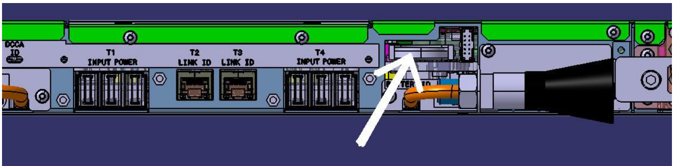
Figure 2 Battery Location with Blue Battery Cover Removed
