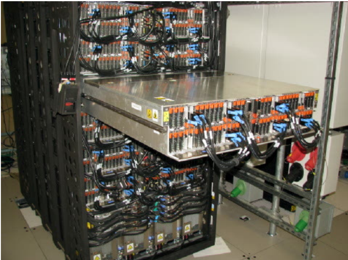
Figure 31 Photo of Disk Enclosure in service position
