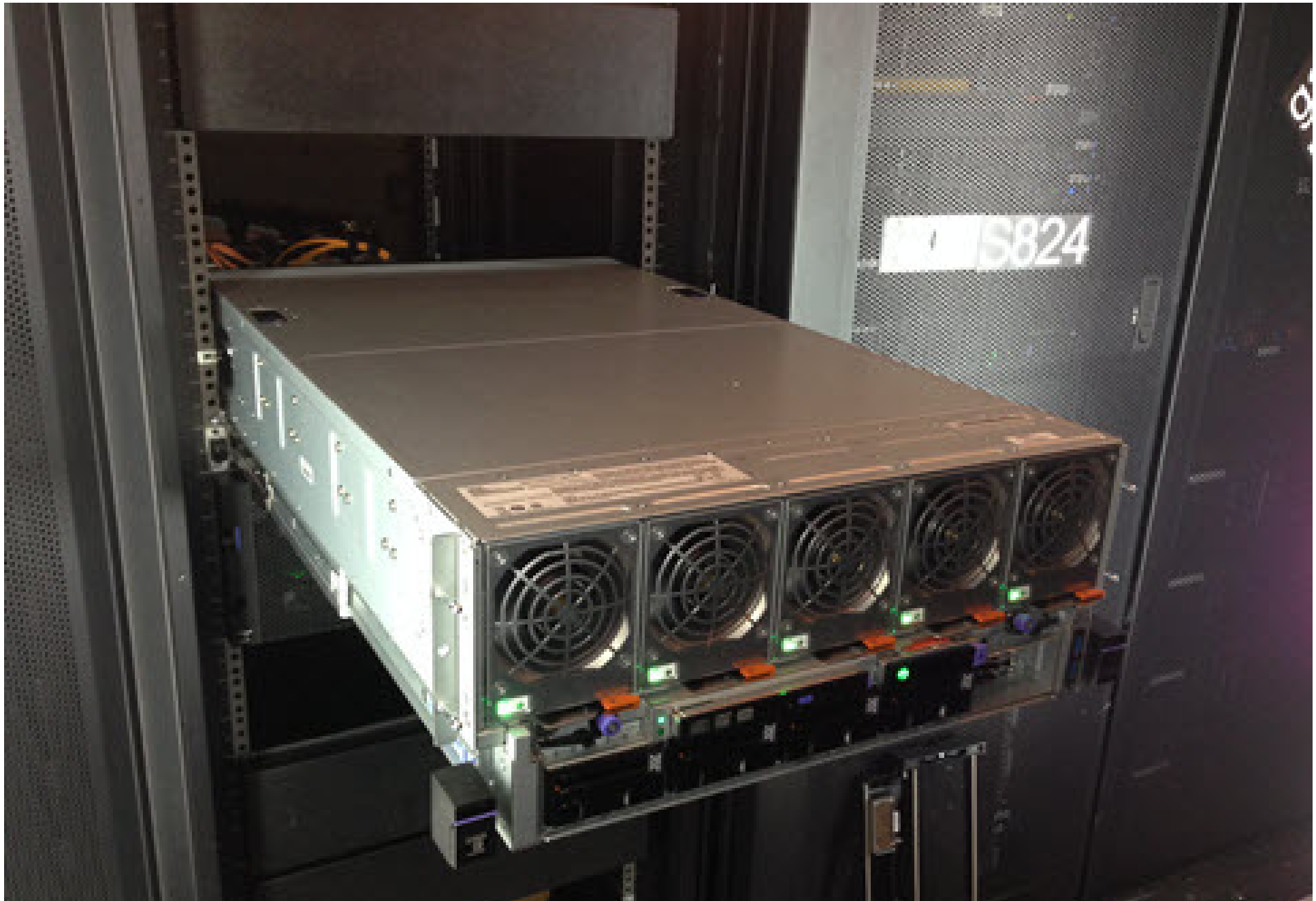
Pulled out of the rack
