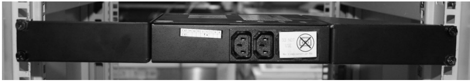
Figure 7. Positioned in rack
