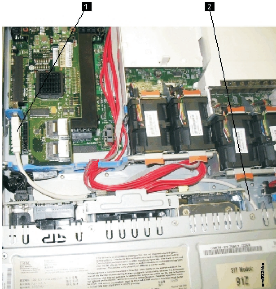
Figure 80. USB service-controller cable connected to the disk controller and USB riser card in the SAN Volume Controller 2145-CF8
