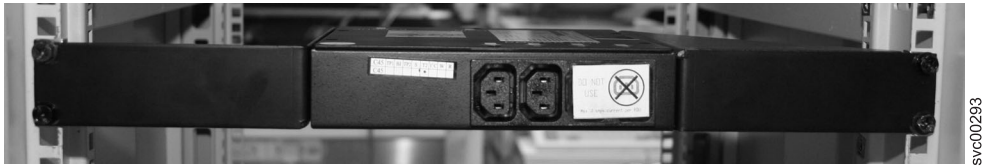
Figure 26. Positioned in rack
