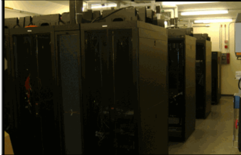
Figure 4-13 IBM GTS scalable modular data center
