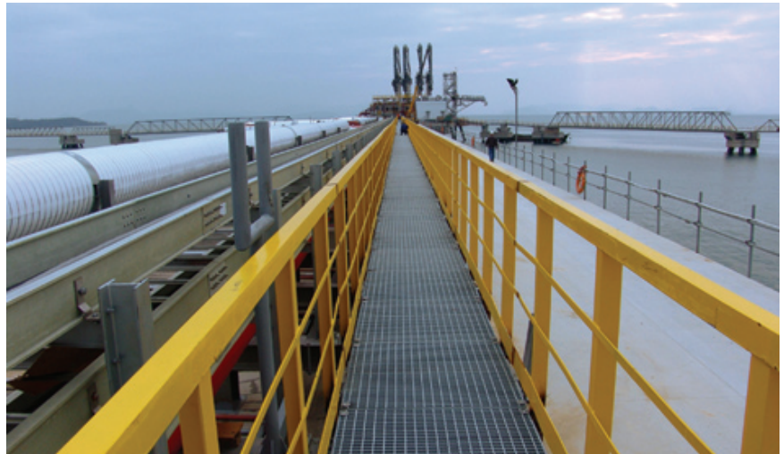
The LNG project of Guangdong Dapeng LNG Company Limited ("DPLNG"), the first of its kind in China, addresses the whole process of LNG import, storage, re-gasification and transmission in China's Guangdong Province. Some of DPLNG's main clients and consumers are the fast growing cities of Shenzhen, Dongguang, Guangzhou, and Foshan City.
