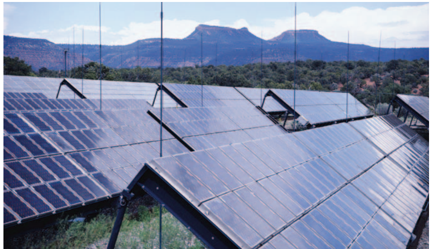
California-based AISO.net has been a trusted name in environmentally friendly Web hosting since 1997. Using solar panels to power its data center and network, AISO.net is the first and only 100 percent completely solar-powered Web hosting company. It currently serves more than 12,000 customers worldwide. AISO.net is the first and only data center in the U.S. to be a member of the U.S. Green Building Council (USGBC).
