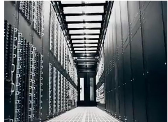
50U tall racks in a data center hall
