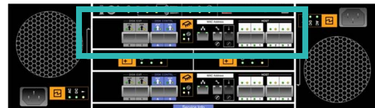
Server Enclosure – Rear
